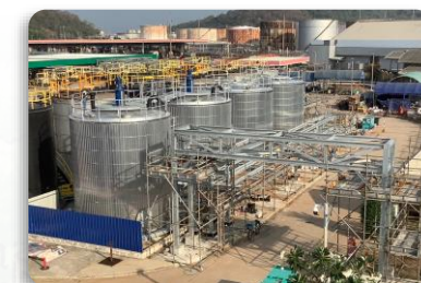
Asphalt AC40/50 Blending plant
