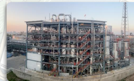
Sustainable Aviation Fuel Unit
